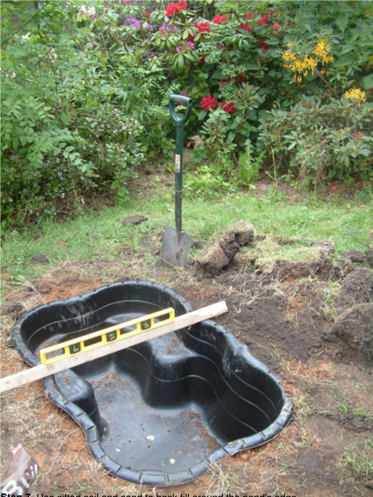
Step 7. Use sifted soil and sand to back fill around the pond's edge
