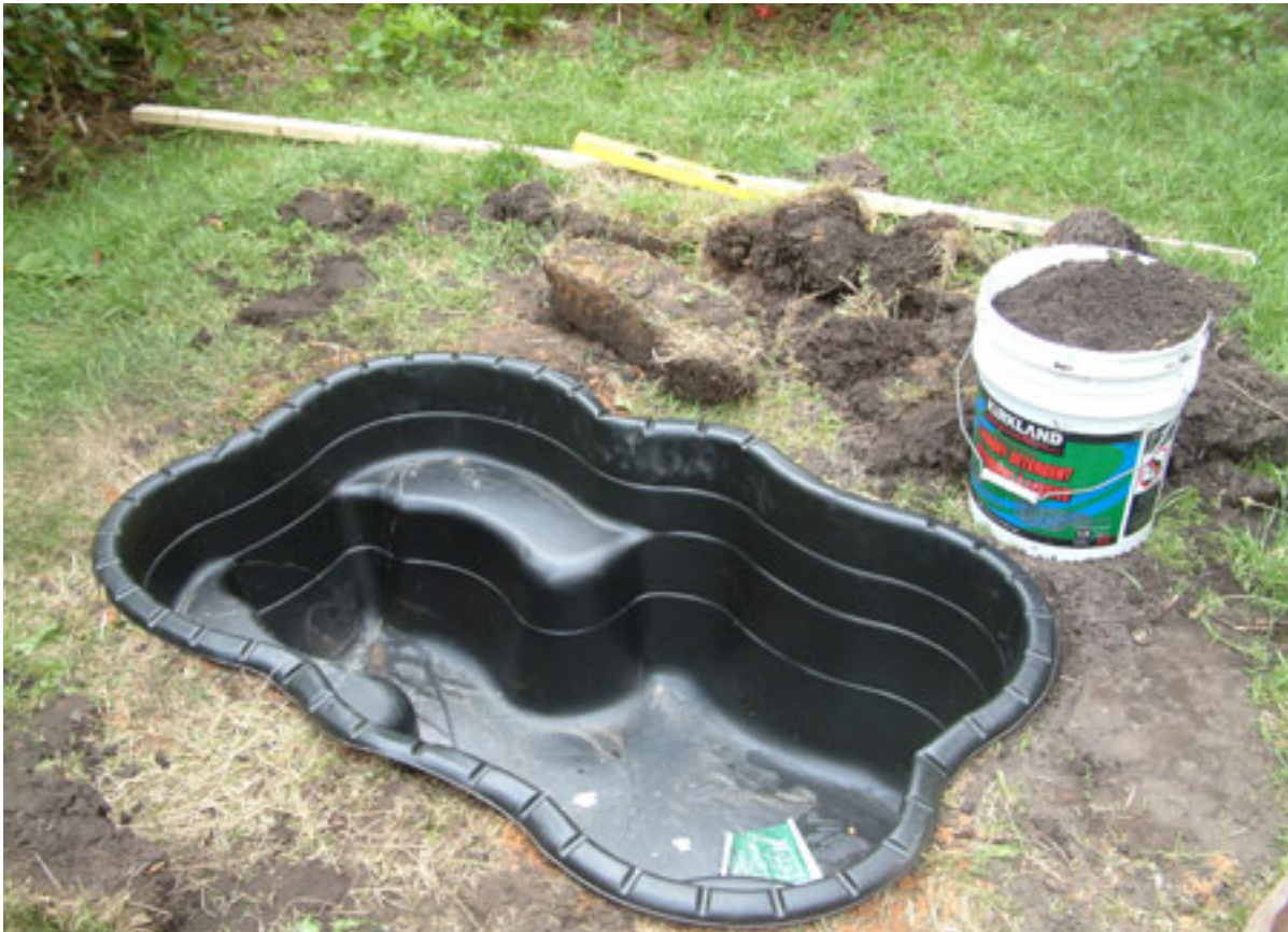
Step 8. Once level, use sand to line the pond and shelves to provide firm support to the pond
