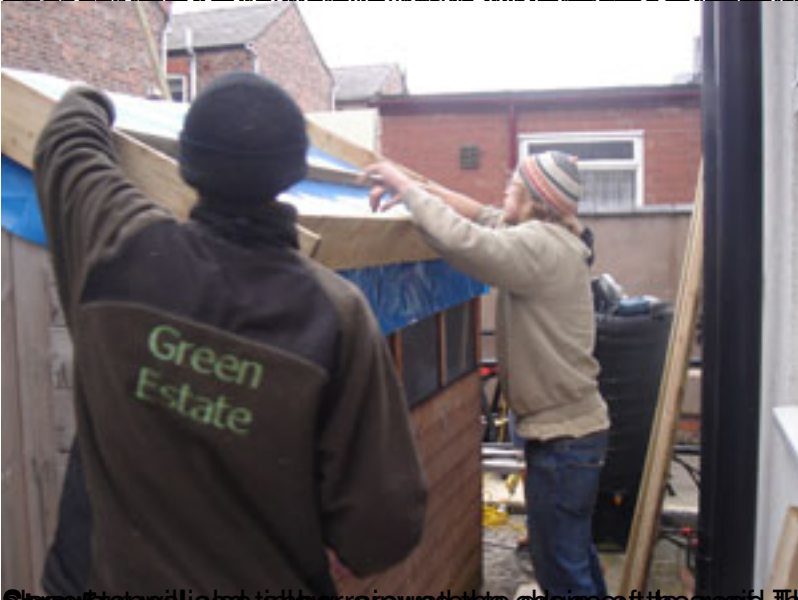
Step 2: The tarp is secured to the roof. The wooden planks are used to support the tarp.
