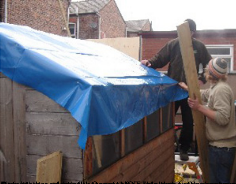
Step 1: The tarp is pulled over the roof. Use existing roof joists to support the tarp.
